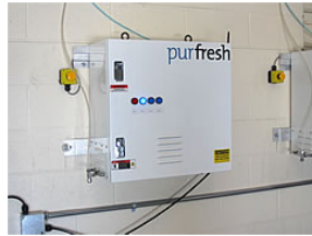
A Purfresh cold storage unit is installed, continuously releasing low concentrated doses of ozone to keep grapes fresh. The technology, says Fremont, Calif.-based Purfresh Inc., is a safer alternative to chemicals such as sulfur dioxide.
